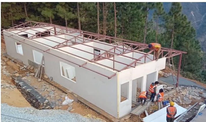
Ongoing construction of panel based Medical Camp Kit (MCK) at Ghetma Health Post, Aathbiskot Municipality
